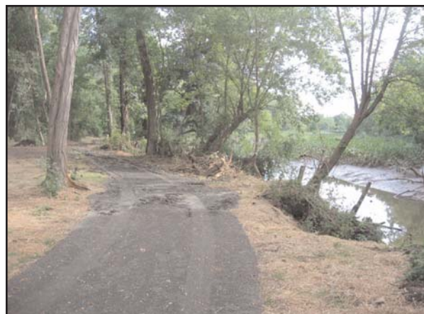
Construction of towpath, with D&R Canal to the right, near remains of Lock #1
